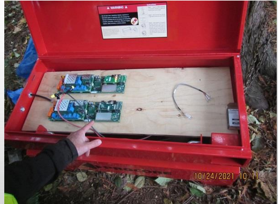
Data collectors and power source for antenna arrays
